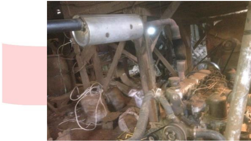
Gambar 2. Kondisi Exhaust System
