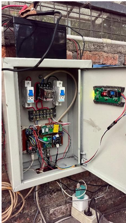
GAMBAR 5 (A). Wiring Kontrol Panel
