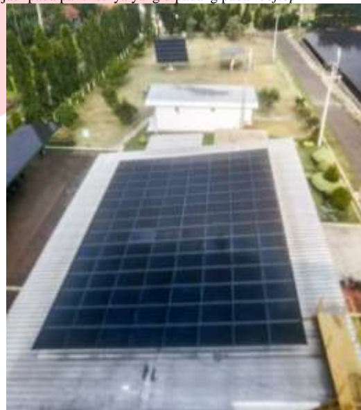
Gambar 4. 7 Rooftop Terkena Shading
