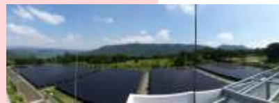
Gambar 3. 5 Array 31 (Ground Mounted)
