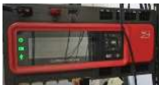
Gambar 3. 3 Data Logger (SMA CLUSTER CONTROLLER)
