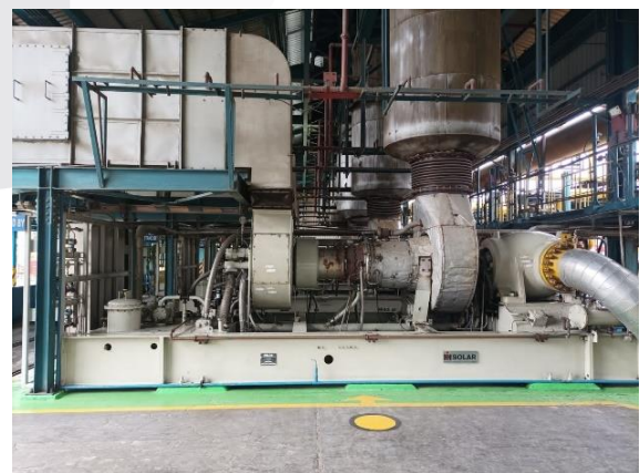
GAMBAR 2 Mesin Gas Gas Turbine Compressor
